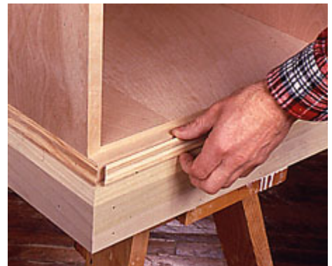
9--Install the baseboard around the desk, then finish the profile by nailing panel molding above the baseboard.
